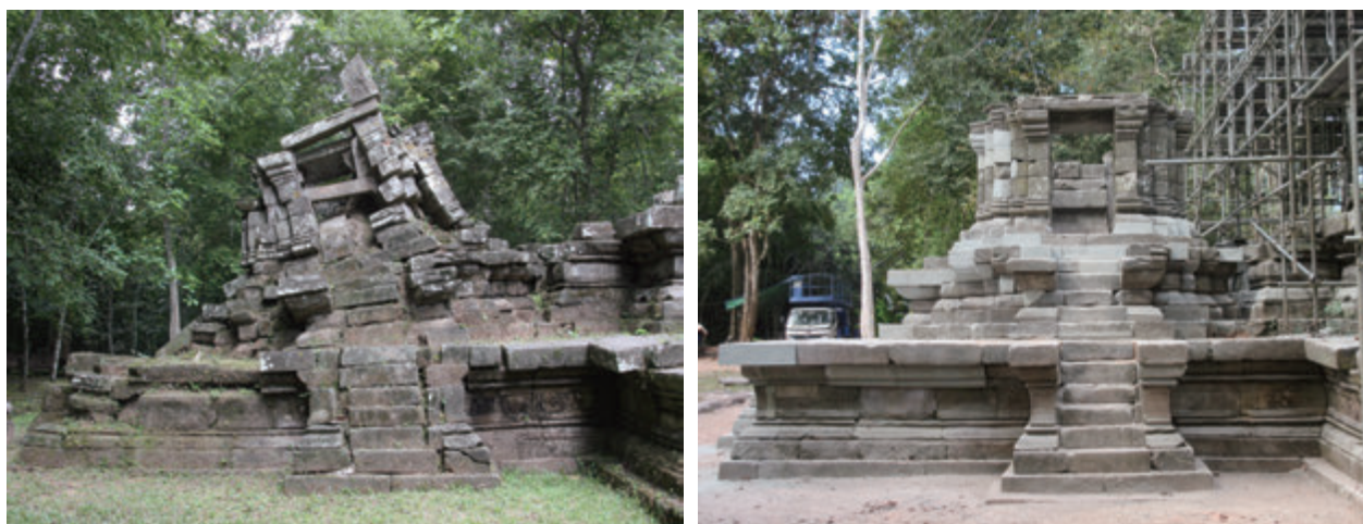
Fig. 2 South sanctuary before the reconstruction (left side), after the reconstruction(right side) (view from the east)
