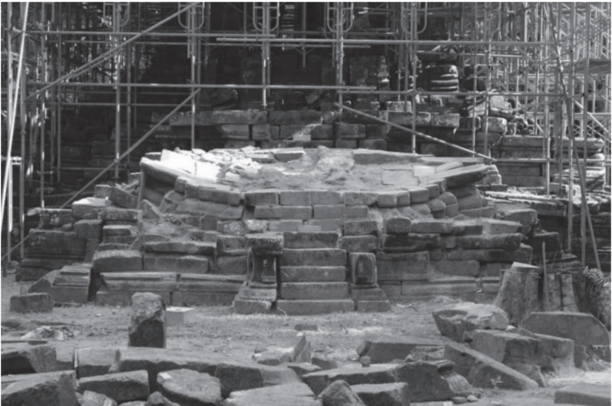
Photo 4: Subsidence of the top surface of the upper foundation
