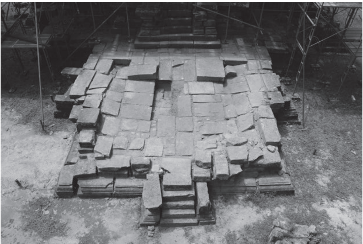
Photo 5: Subsidence of the paving stones on the surface of the lower platform
