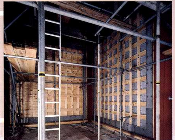
Inside the walls for the first story (Strengthened with wooden frames and metal fittings)
