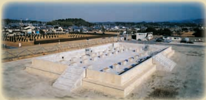
After protecting the archaeological features with a layer of fill, the podium was built without using any stakes. Seismic dampers were employed within the podium to lessen the force of earthquakes.
